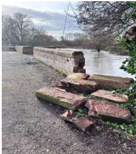
New flood debris damage to arch parapet, 18 November 2025
