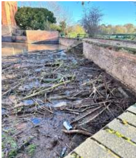
Debris, arches over Powick Mill Pond, 15 November 2025
