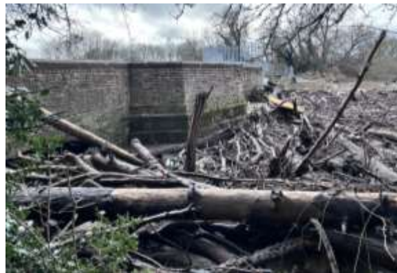
On-going flood debris build-up 30/1/2026
