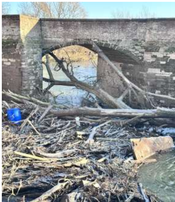
Flood debris build-up 31/12/2025
